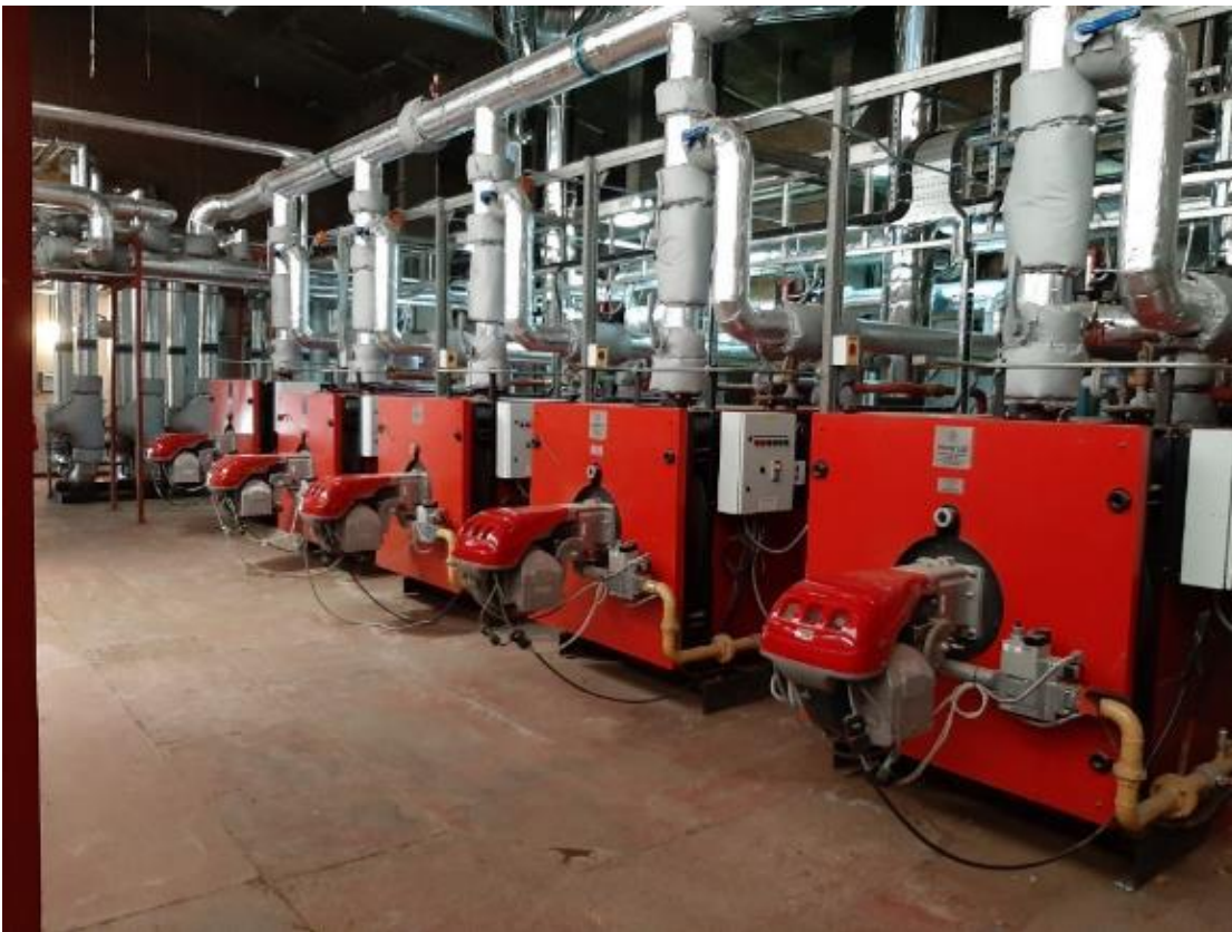
Figure 15: Broadwater Farm boiler location – new and refurbished boilers and pipework. This photo shows the red boilers and their pipework in the newly referbished boiler house.
