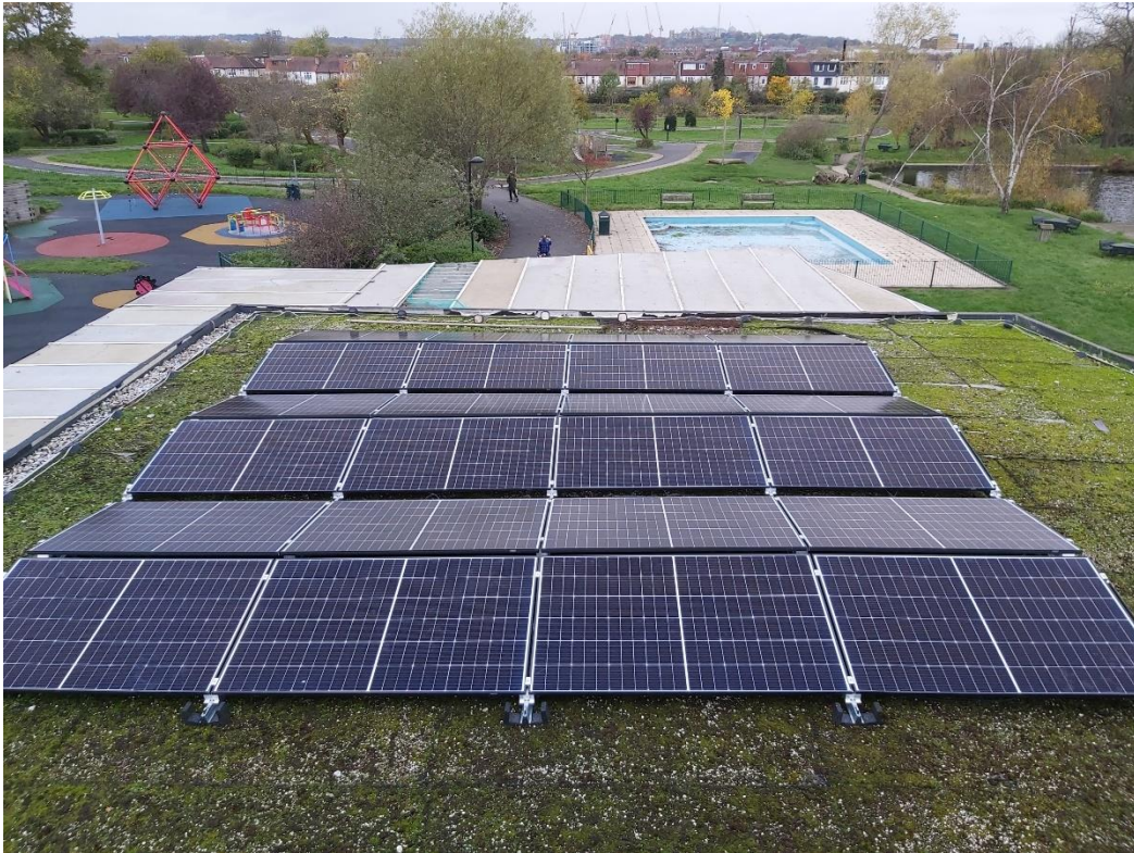
Figure 20: Solar photovoltaic panels installed on the roof at Lordship Hub in November 2022.
