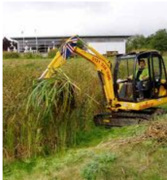
Hopwood Park MSA M42. A light tracked excavator removes aquatic vegetation to de-water next to the wetland, before moving to a wildlife pile.
