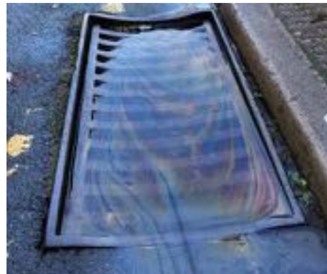
Pollution from roads and car parks is often visible - fuels, oil, heavy metals, tyre dust and silt all get washed into drainage systems.
