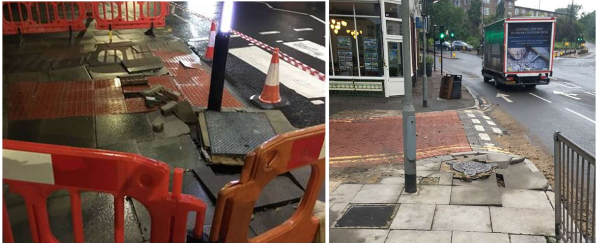
Figure 5-5 Pavement damage, Cranley Gardens and Etheldene Avenue
