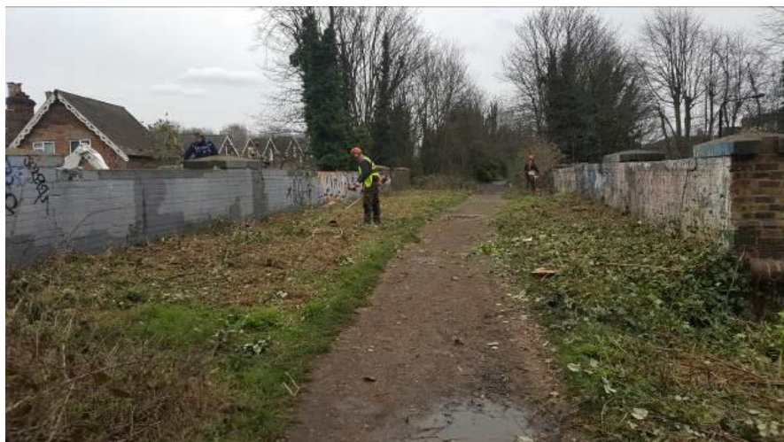
Image 20: Vegetation clearance to enable bridge inspections in advance of major repair works
