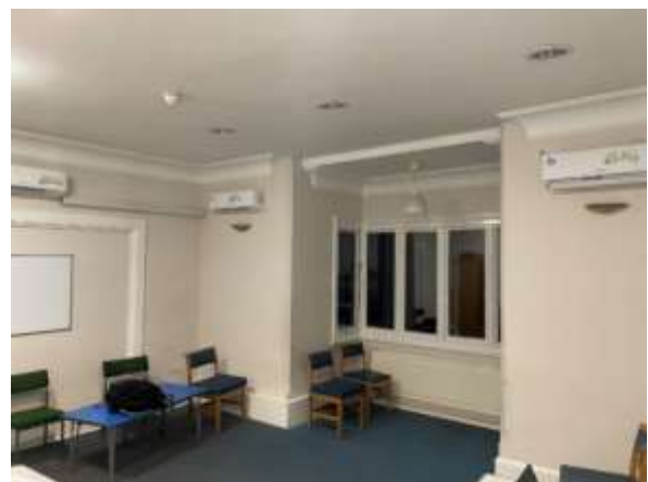
Figure 25: The Holly meeting room at Muswell Hill Methodist Church, heated by the part-funded air source heat pump. The heat pump is located on the roof outside of a side elevation of the hall.
