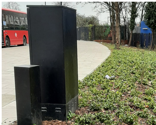
Utility cabinet – Tottenham Hale
