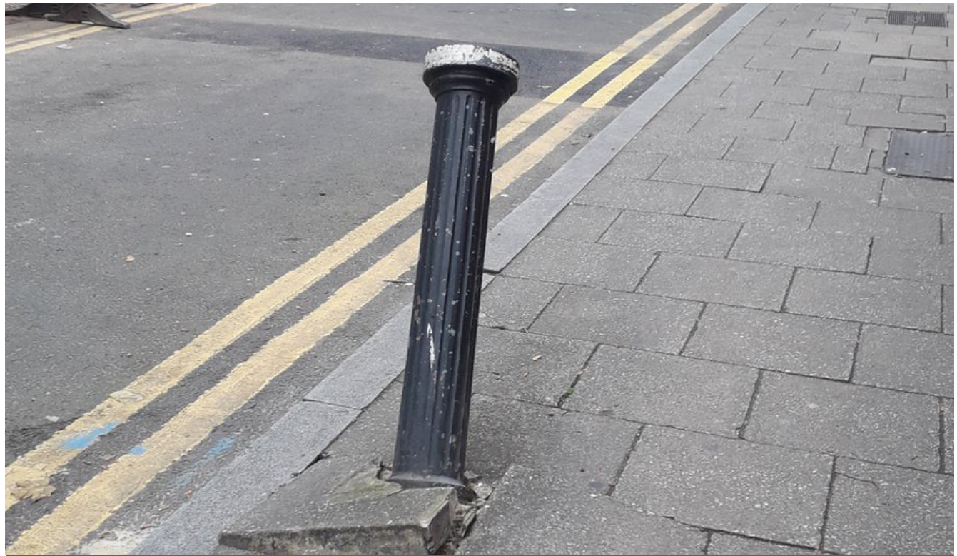
Furniture causing accessibility issues
