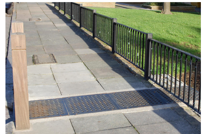
Drainage gully - Boyton Road
