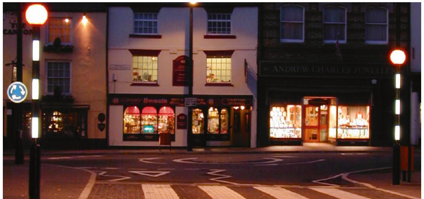
Pedestrian crossing control unit
