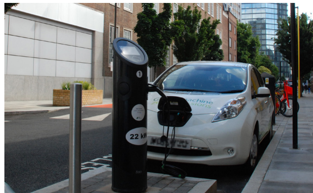
Electric charging point - Moreland Rd, Islington
