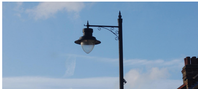
Street lighting – Lordship Lane
