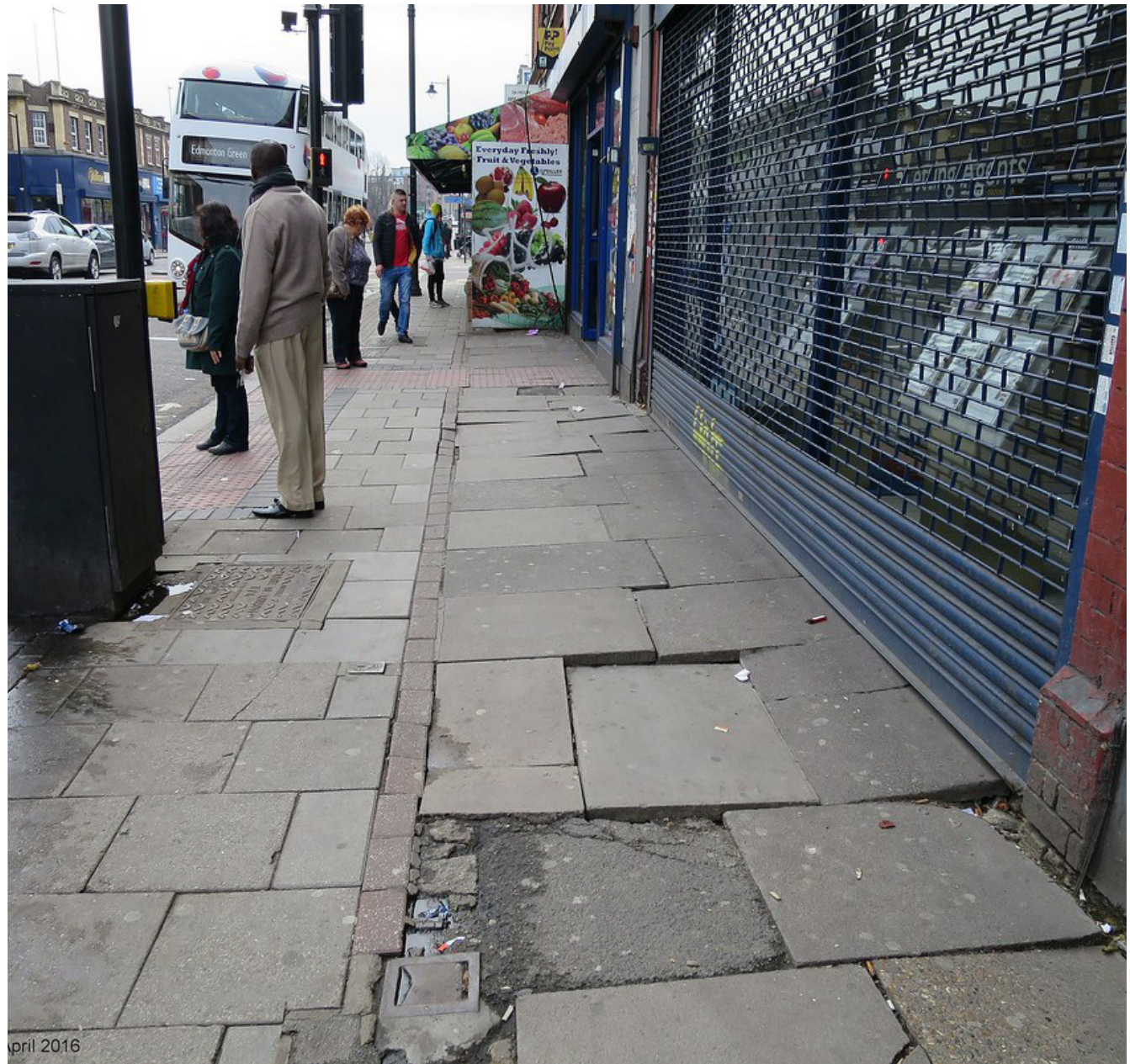
Damaged pavement slabs at 471 High Road - 2015
