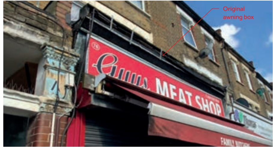
Example of a surviving awning box in Tottenham fitted to the top of the fascia. Original awnings have the potential for repair and re-use. A modern awning has also been fixed to the external shutter box, which increases the depth of the assembly and obscures original detail
