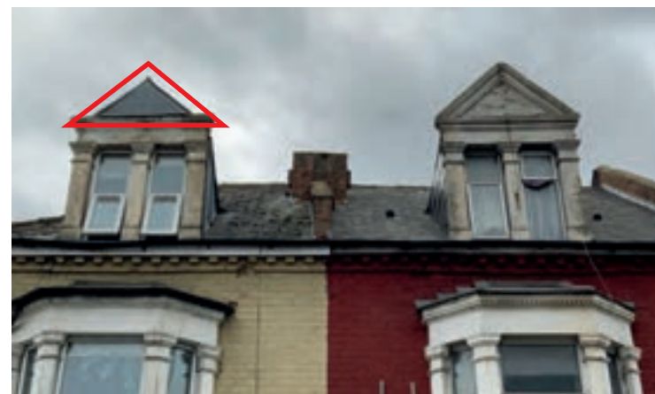
Reinstatement of the top section of the dormer can be based on the surviving details to the adjacent building in Seven Sisters
