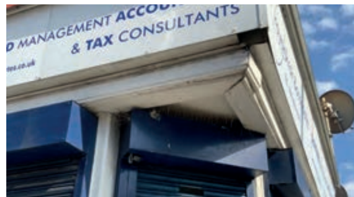
The original cornice, fascia and architrave have been obscured by the modern bulky sign on this shop in Tottenham
