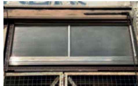
Surviving Art Deco shopfront with stainless steel frame and reeded glass, No 80 Bruce Grove
