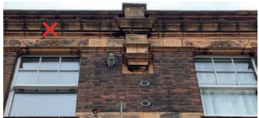
Flues should be in unobtrusive locations that are not visible from the street, in contrast with those shown on this building in Tottenham
