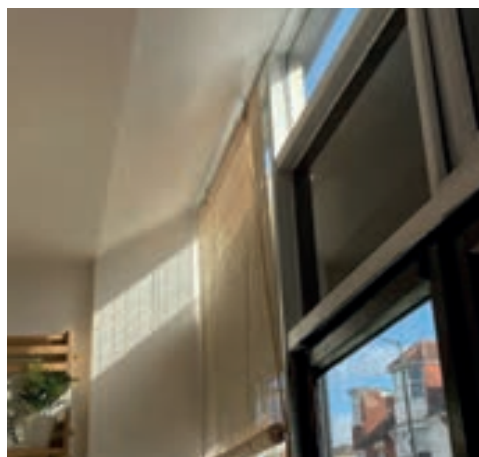
Suspended ceilings should use a splay to avoid obscuring the shop window, as seen here in Tottenham
