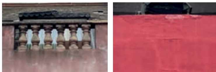
Reinstatement of the missing balustrading would reinforce the link between these buildings and their prominence in Tottenham
