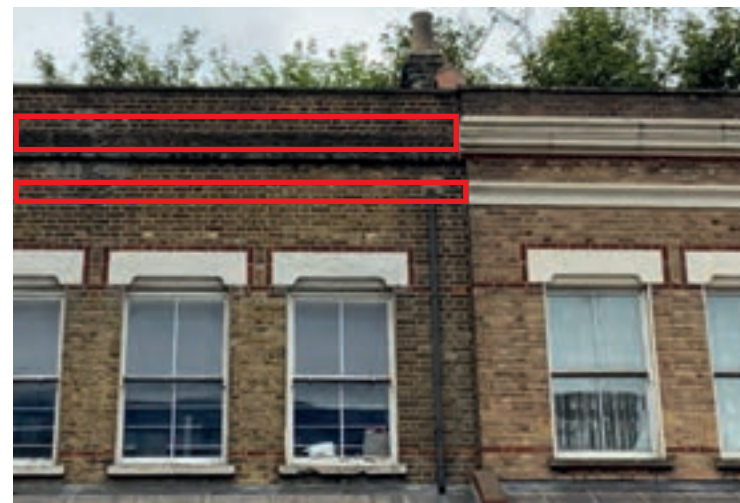
Reinstatement of the missing sections of cornice would complete the terrace and reinforce its status as a local landmark in Tottenham
