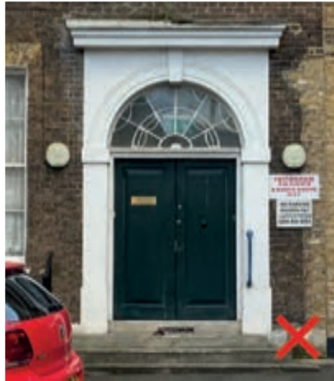
To avoid clutter and potential damage to historic fabric, light fittings should not be fixed to the building façades, as this one on Bruce Grove is
