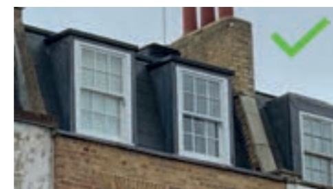
Dormers should be clad with lead sheet or tiles, retaining the original form and scale, as in this example in Highgate
