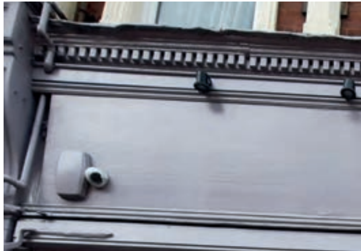
Shopfront with cornice and architrave to define top and bottom edges of fascia (Crouch End)
