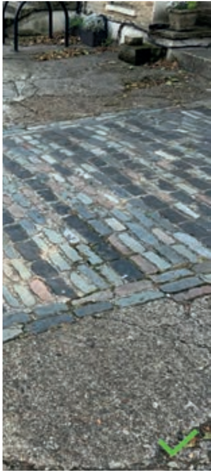
Surviving section of original/early cobbled surfacing to No 16 Bruce Grove that probably related to a former carriage entrance. This can be conserved and replicated on other properties
