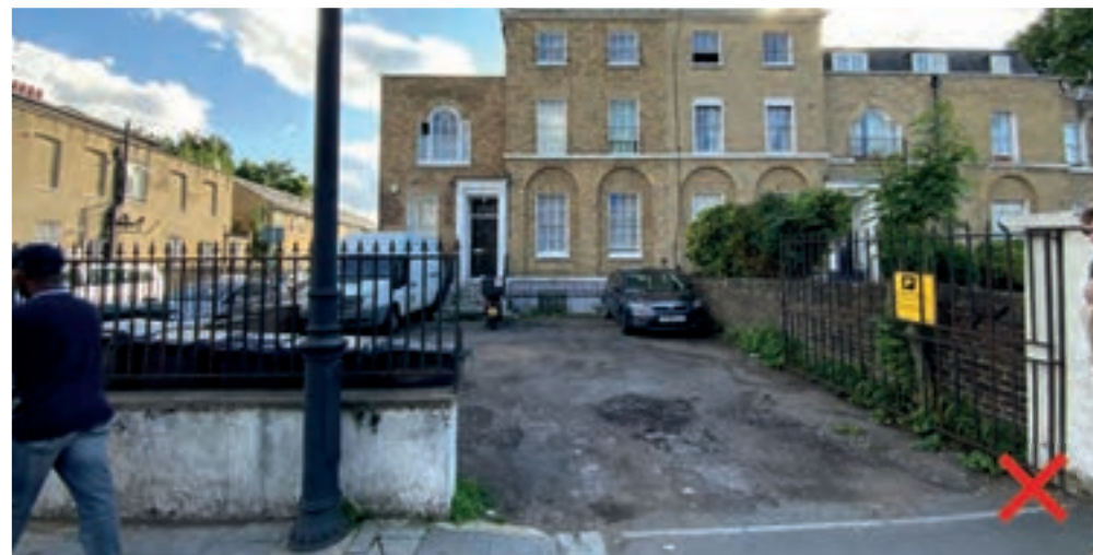
Modern tarmac on Bruce Grove surfacing in varying condition has a detrimental impact on the setting of the listed buildings
