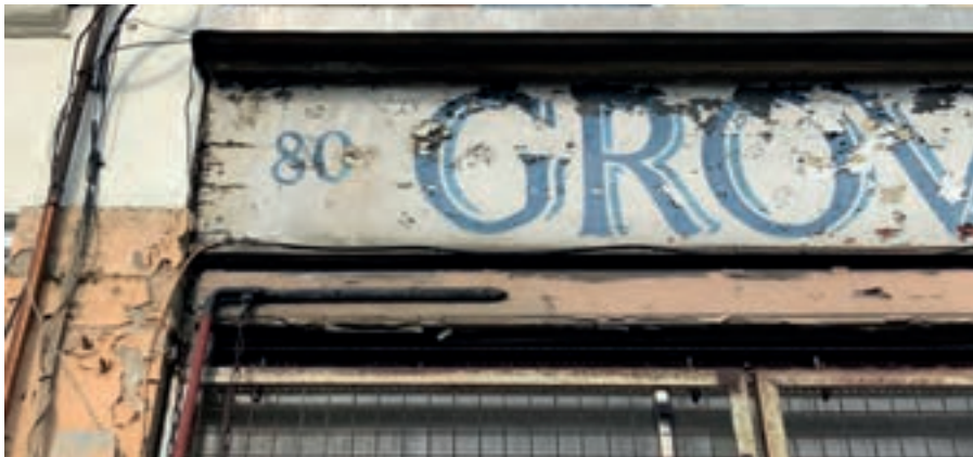
Historic awning in Tottenham, located beneath the fascia with the potential to be refurbished
