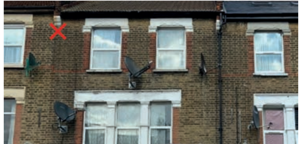
Satellite dishes should not be fixed on the front of buildings, as they are on this building in Tottenham
