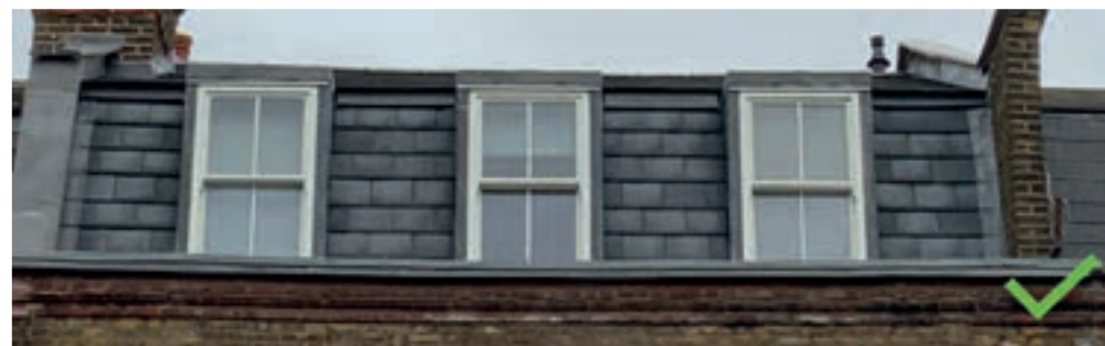
On older buildings, roofing material will generally be natural slate or clay tile, as in this example from Highgate
