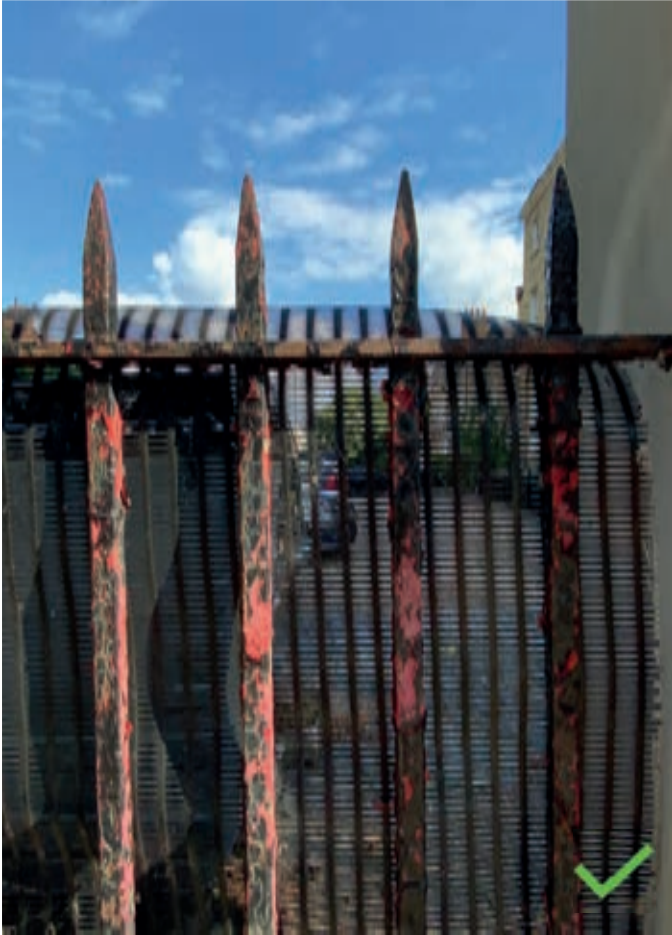
Surviving section of original railings to 16 Bruce Grove, providing a historical precedent for use in other locations. Note that exposed tops to new railings should be flat and not spiked to prevent injury
