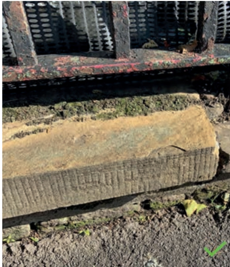
Surviving section of original brick boundary wall to 16 Bruce Grove with York stone copings, providing a historical precedent for use in other locations
