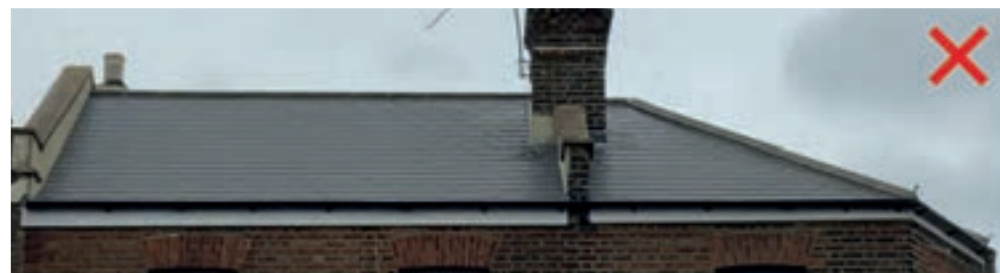
Imitation slates or concrete tiles such as these in Tottenham often appear as 'two-dimensional' replicas
