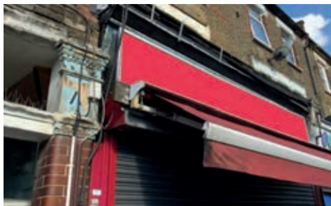
The original awning box and fascia sign have been neglected in favour of a new sign and blind which obscure original fabric and add a bulky profile to this shopfront in Tottenham
