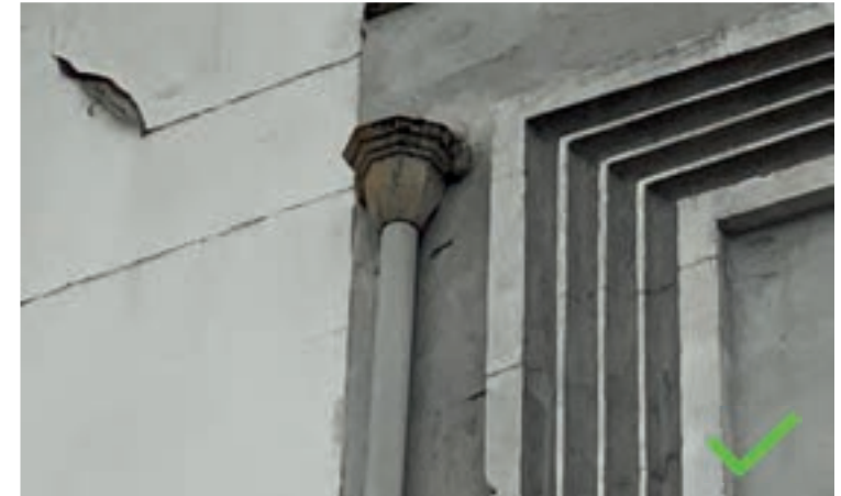
Where present, surviving historic cast-iron hoppers, such as this one in Tottenham, and rainwater pipes should be retained and refurbished
