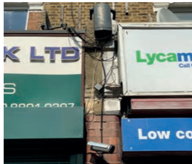
Services should have concealed pipe and cable runs and be located in unobtrusive locations that do not obscure original detail, as this service installation in Tottenham does
