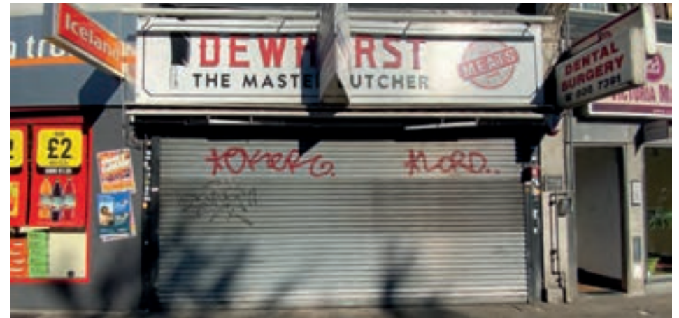
Solid external shutters obscure views of window displays and have a deadening effect on the street whilst providing a canvas for graffiti, as seen here in Tottenham
