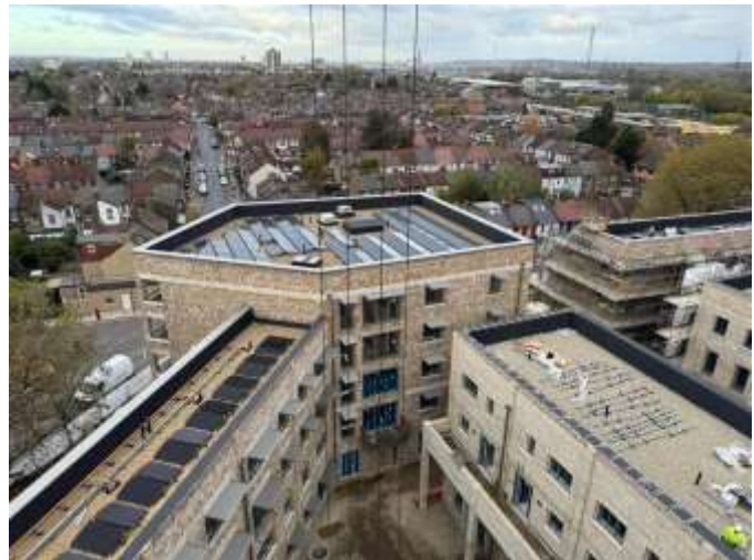
Figure 10: Image showing part of the Ashley Road development from above, with external shading, and solar PV being installed onto roof spaces.
