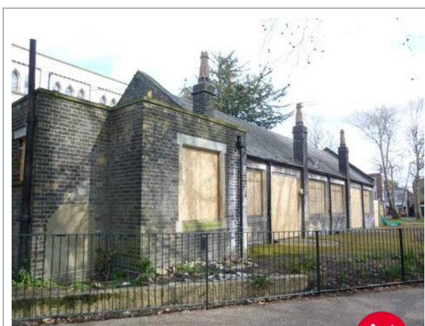
Examples of buildings in Bruce Grove and Tottenham Green Conservation Areas that have fallen in to disuse can be in danger of neglect.
