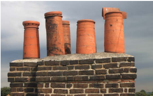
Handmade chimney pots – one is to be replaced.
